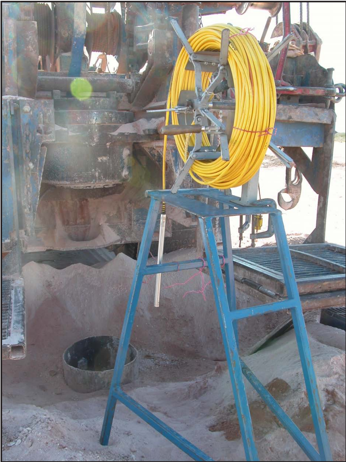
Figure 3-2. MiniTroll being set up at SNL-13 on April 11, 2005 to monitor Dewey Lake water.
